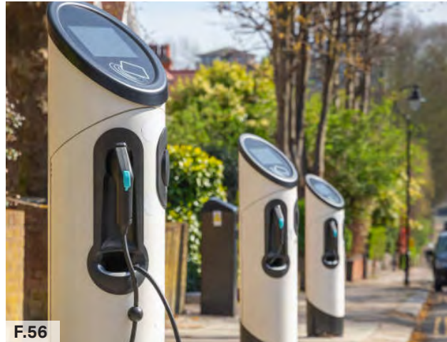
Figure 56: Examples of on-street car charging points.
