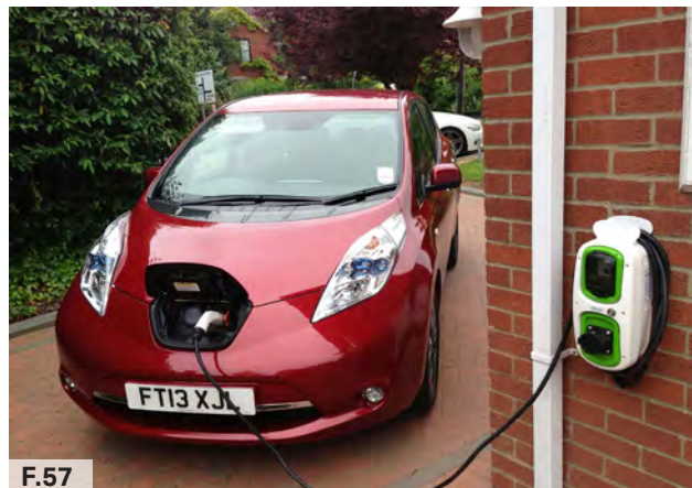
Figure 57: Examples of off-street mounted car charging points.
